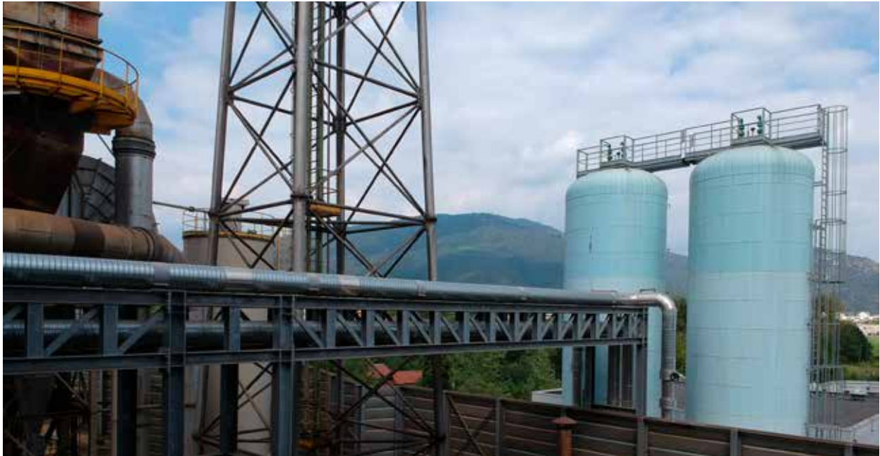
Alfa Acciai: array of pipes supplying the heat recovery plant from the steel mill and storage tanks
